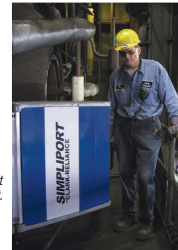
100 year old power plant with Simpliport retrofit.
